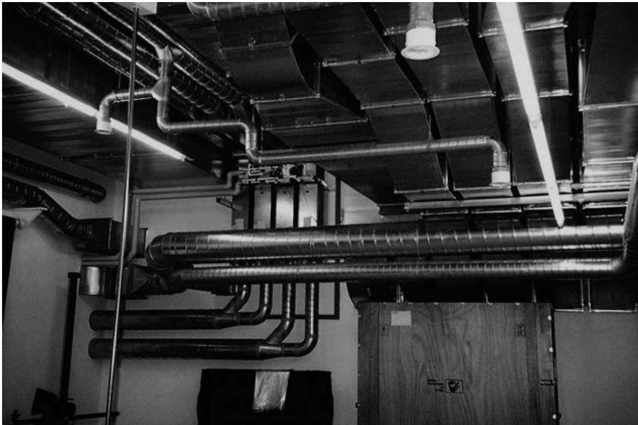
Partial view of the air-conditioning system of the Fondation Beyeler Museum in Rieten, near Basel, by Renzo Piano, 1997.
